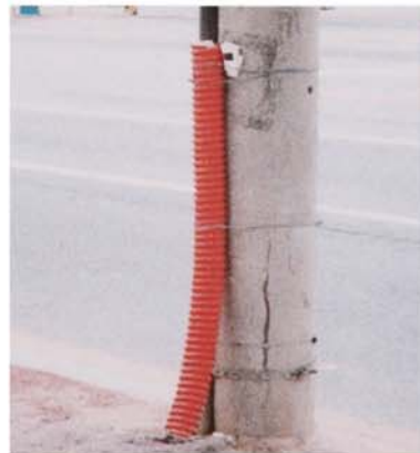
▲ Inlet of cable form pole.
